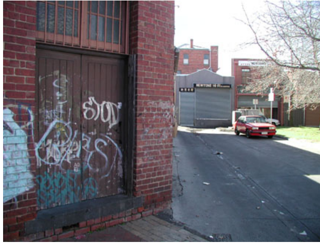
Figure 16: Location requiring graffiti removal
